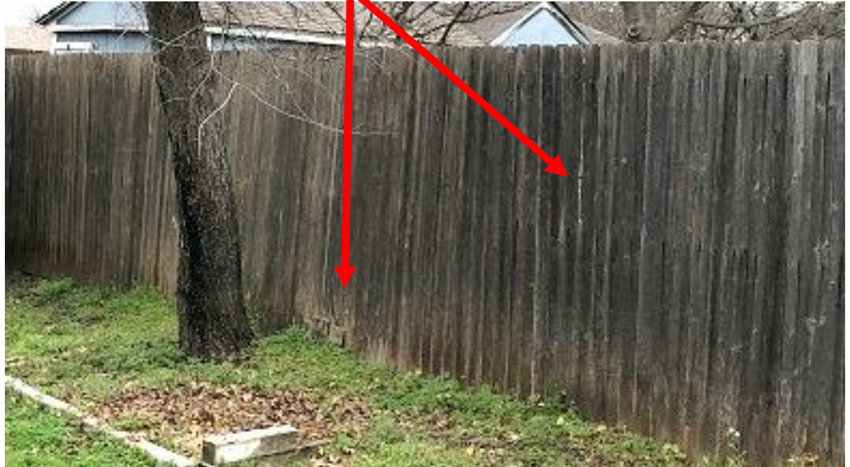
7 Fence with warped and rotting pickets
